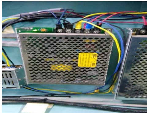
Figure 7. Power Supply 12VDC no output
