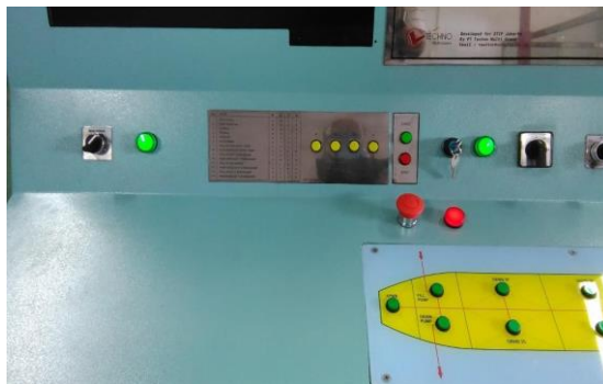
Figure 8. Install Key switch + green indicator to activate the Actuator when it is operated and Emergency switch + red indicator for emergency stop in the event of a malfunction the actuator moves outside the control command.
